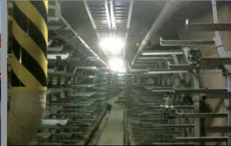
Prague City Utility Tunnels, Czech Republic
