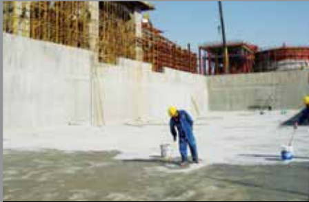
Coal Storage at Power Station, China
