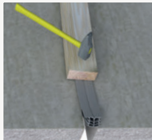
The profile is then pressed into the joint with the help of wood facing.
